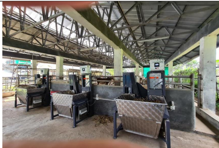
One unit of greenfeed and three units of Smartfeed Pro has been installed at Indonesian Research Institute for Animal Production (IRIAP) at Bogor West Java
