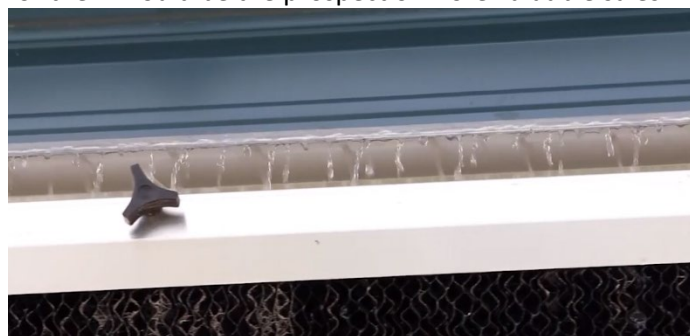
Picture: 1: Large pig production unit cooling system
