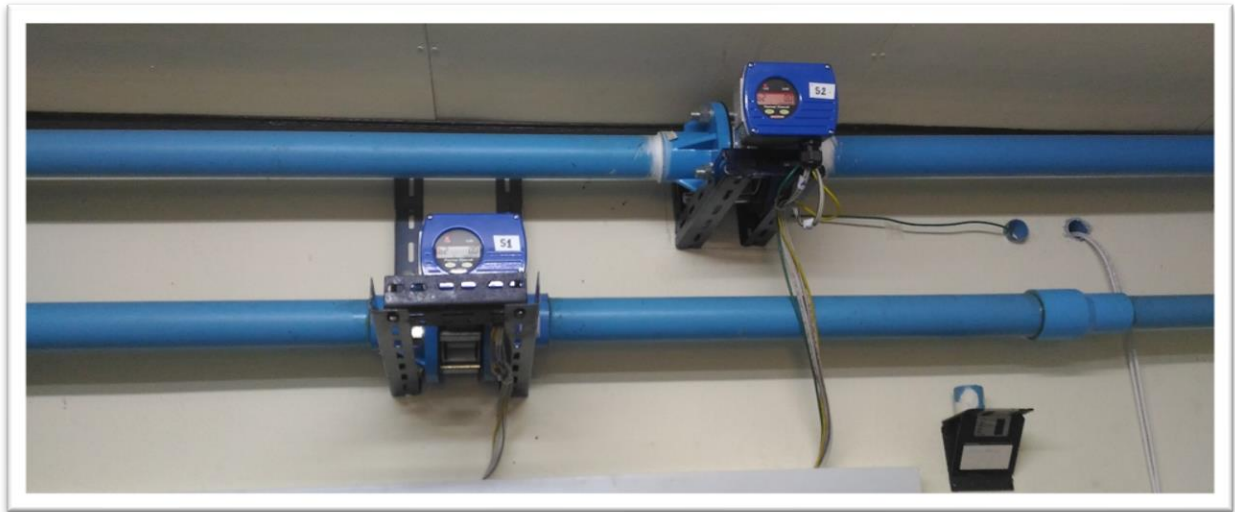
Fig.7 Flow meter and main air tube
