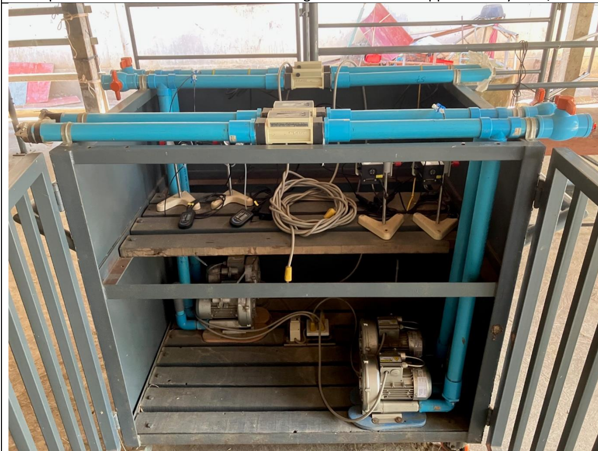
The core of the headbox system is the mobile airflow and analysis hub. This system can be closed off for security but in it is housed 4 side-channel blowers (on floor of box) connected to the 4 air flow ducts (blue pipe) running along the top), which have a "t" piece junction and a ball-type valve to allow outside air into the blowers and thus reduce the amount of air drawn from the headboxes. Fitted into the air flow system across the top of the trolley are 4 turbine flow meters. Narrow diameter tube samples air from each the 4 blue pipes and this air is pumped by a 4 mini peristaltic pumps (seen with V shaped stands on middle level) and into a tedlar gas collection bag (not shown)
