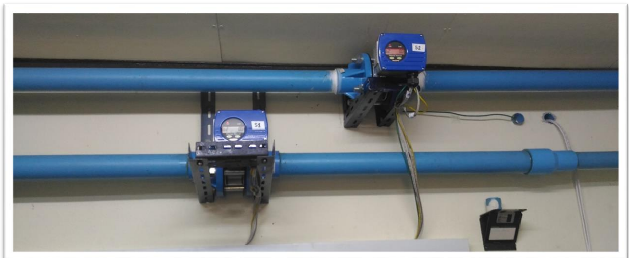
Fig. 7. Flow meter and main air tube
