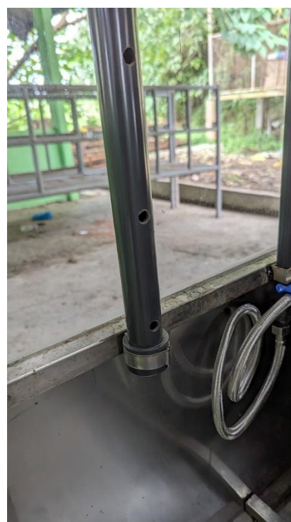
f. Vertical 1-inch pipes with holes for the entry of air to be analyzed
