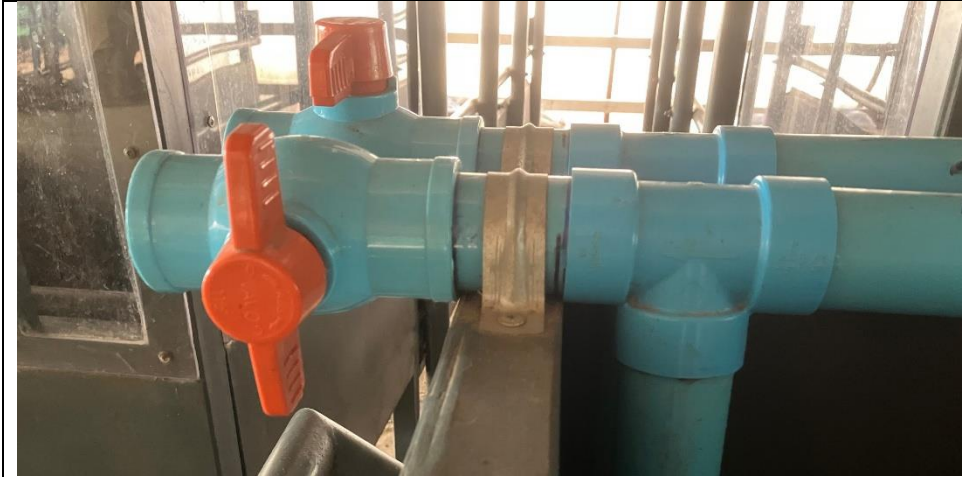
Ball valve that allows the balance of air drawn from the he4abdox and from the outside atmosphere to be varied to ensure flow through the headbox is approximately 500L/min
